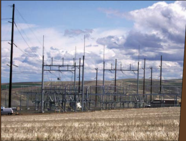
Talbot Substation Dayton, Washington
